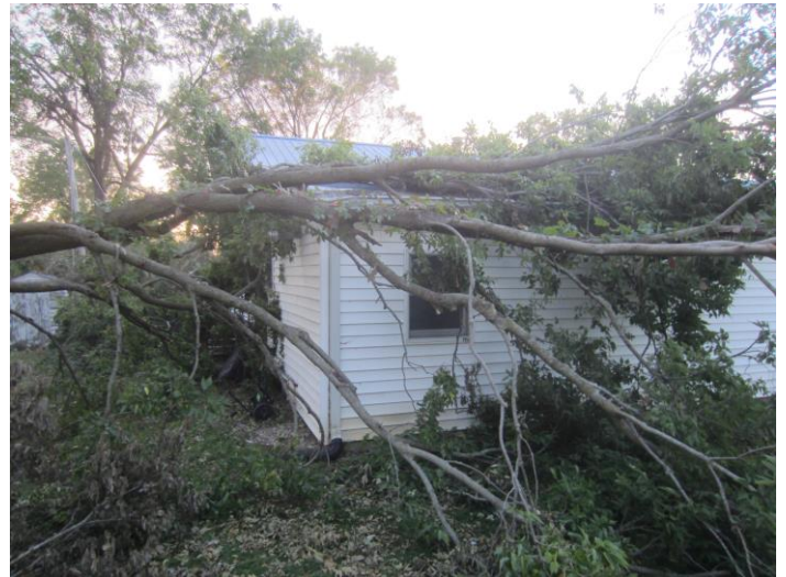
Damage to the SW corner of the building
